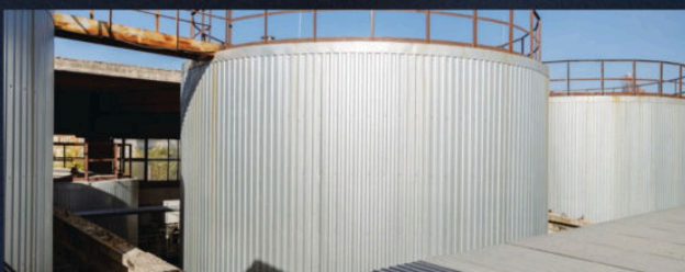
CPO STORAGE TANK
